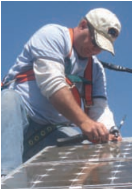
Electricians have an obvious advantage when it comes to solar, but still need training on solar system design and working with high-voltage direct current.
